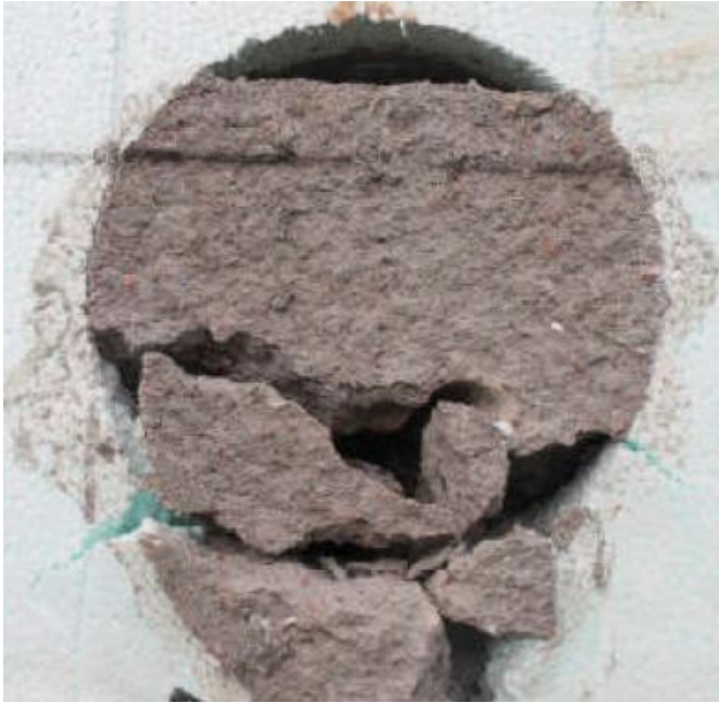
Anchor installed off-centre
